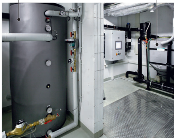
Stratified storage tank
